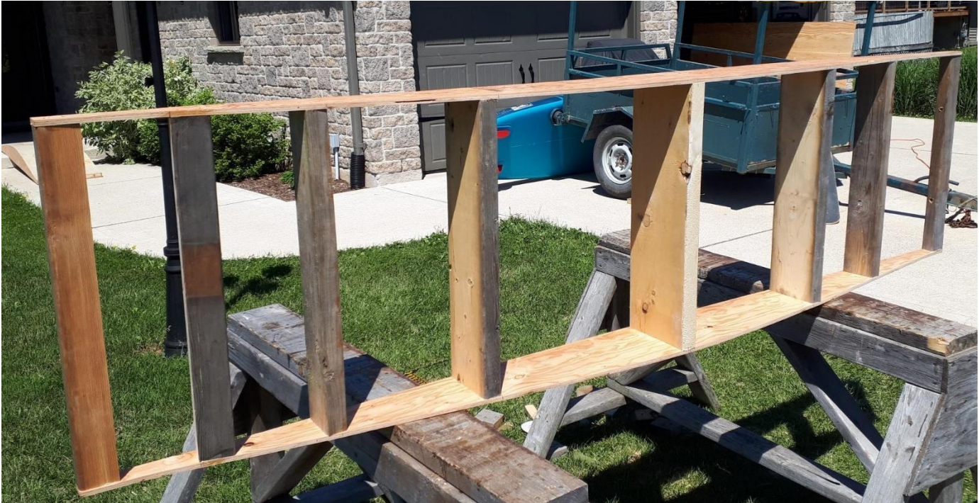
Figure 6. Placement of 2x6 and 2x4 principal joists. Note that this is an end section. The left side of this section is an entrance/exit. The 2x4 joist is placed on edge to maximize the surface area available to join in the end ramp boards. (refer to previous Figure 4).
